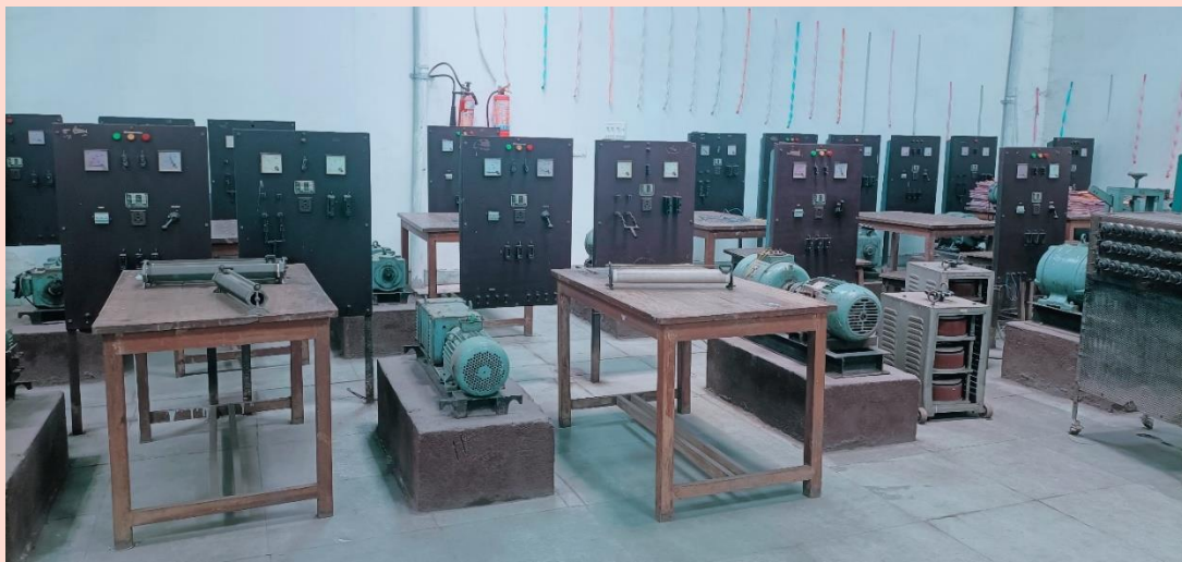
Electrical Machine Laboratory
